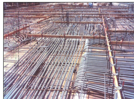
Fig. 1: An example of the congestion of conduits in a slab
