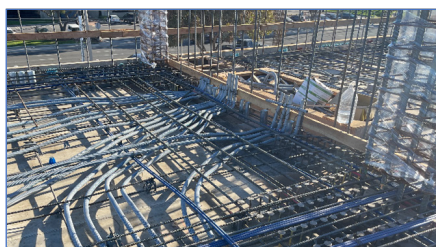
Fig. 4: A close-up of the reinforcement at the edge of a shear wall to be cast where the vertical bars at the right of the image are (photo taken in 2024). Note from the shadows on the conduit that many of these appear to be within 1 in. or less of the top reinforcing bar curtain in the slab
